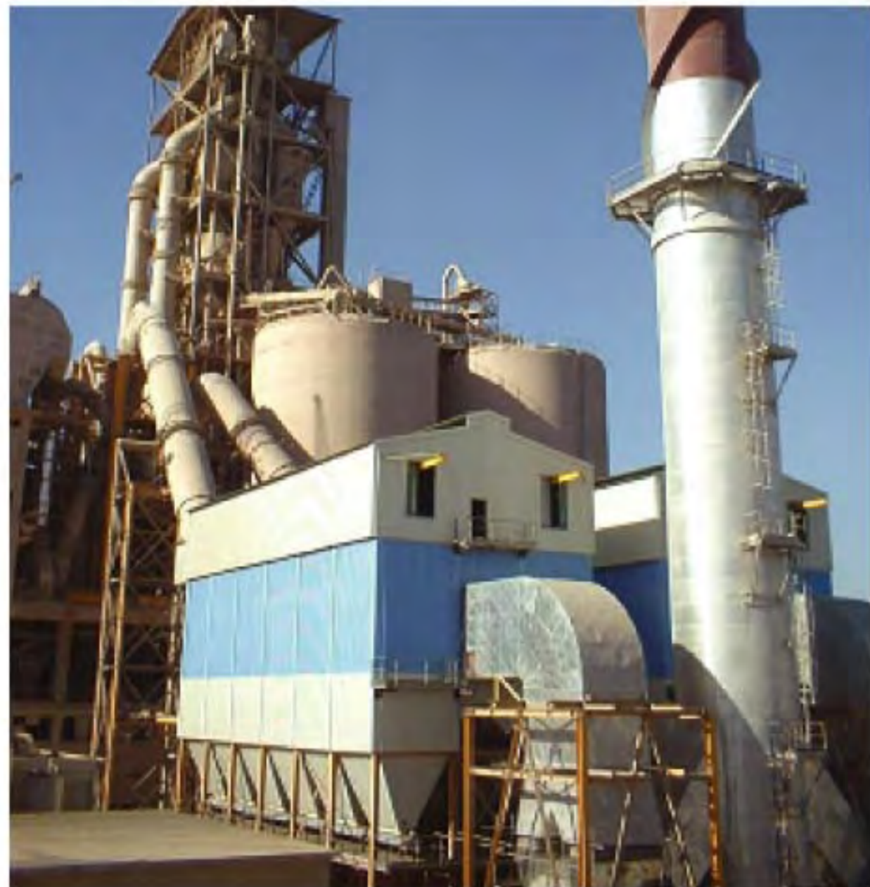
AAF Fabri-Pulse XLC bagfilter controlling emission for Preheater kiln and raw mill in a cement plant at Algeria.
