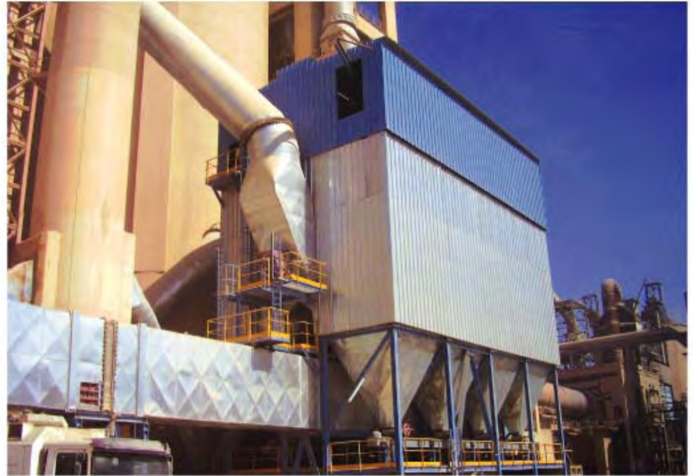
Fabri-Pulse XLC Filter for Kiln & Raw Mill in Tunisia.
