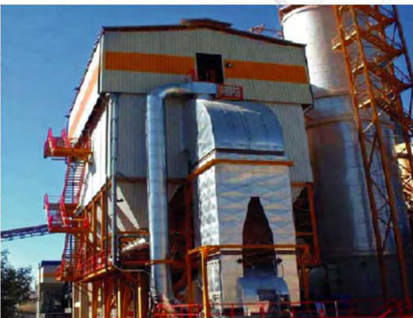
CIMPOR, Portugal. Fabri-Pulse XLC Filter for Kiln & Raw Mill
