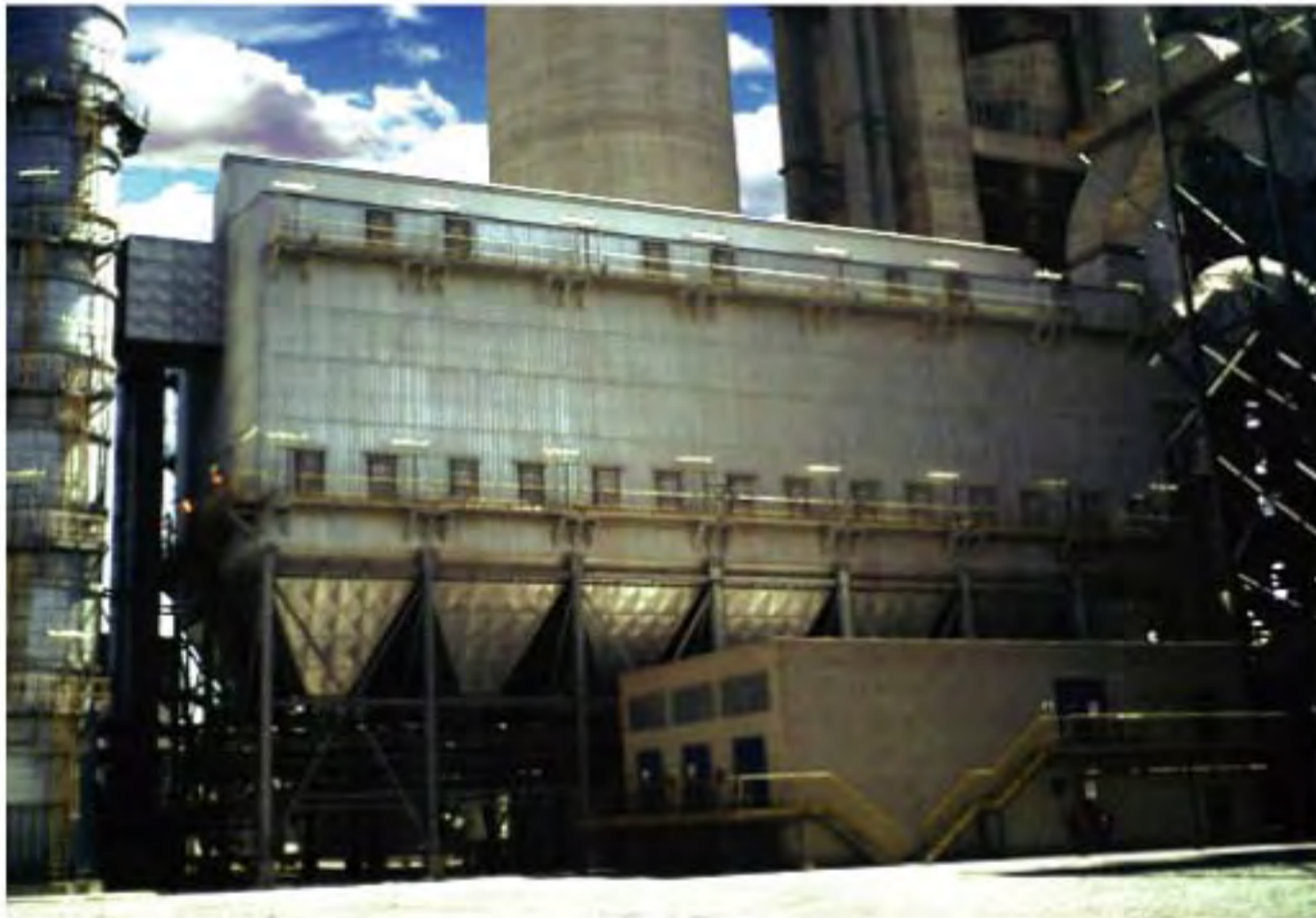
Amer-Therm Reverse Air Filter for Kiln & Raw Mill in Argentina.
