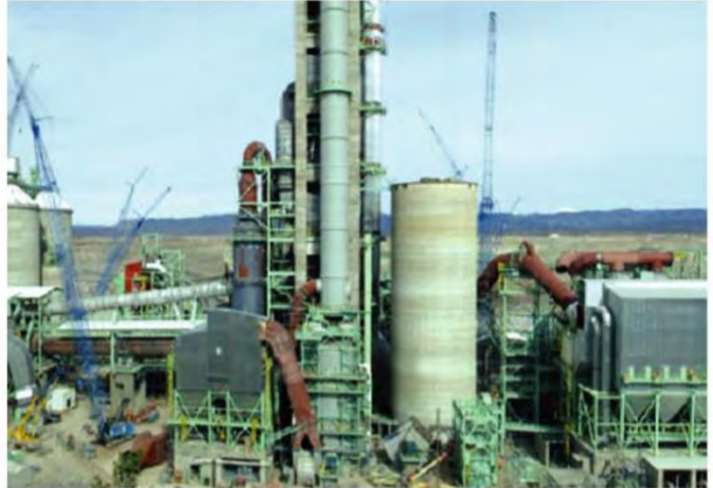
HOLCIM, United States. Fabri-Pulse for Alkali Bypass.
