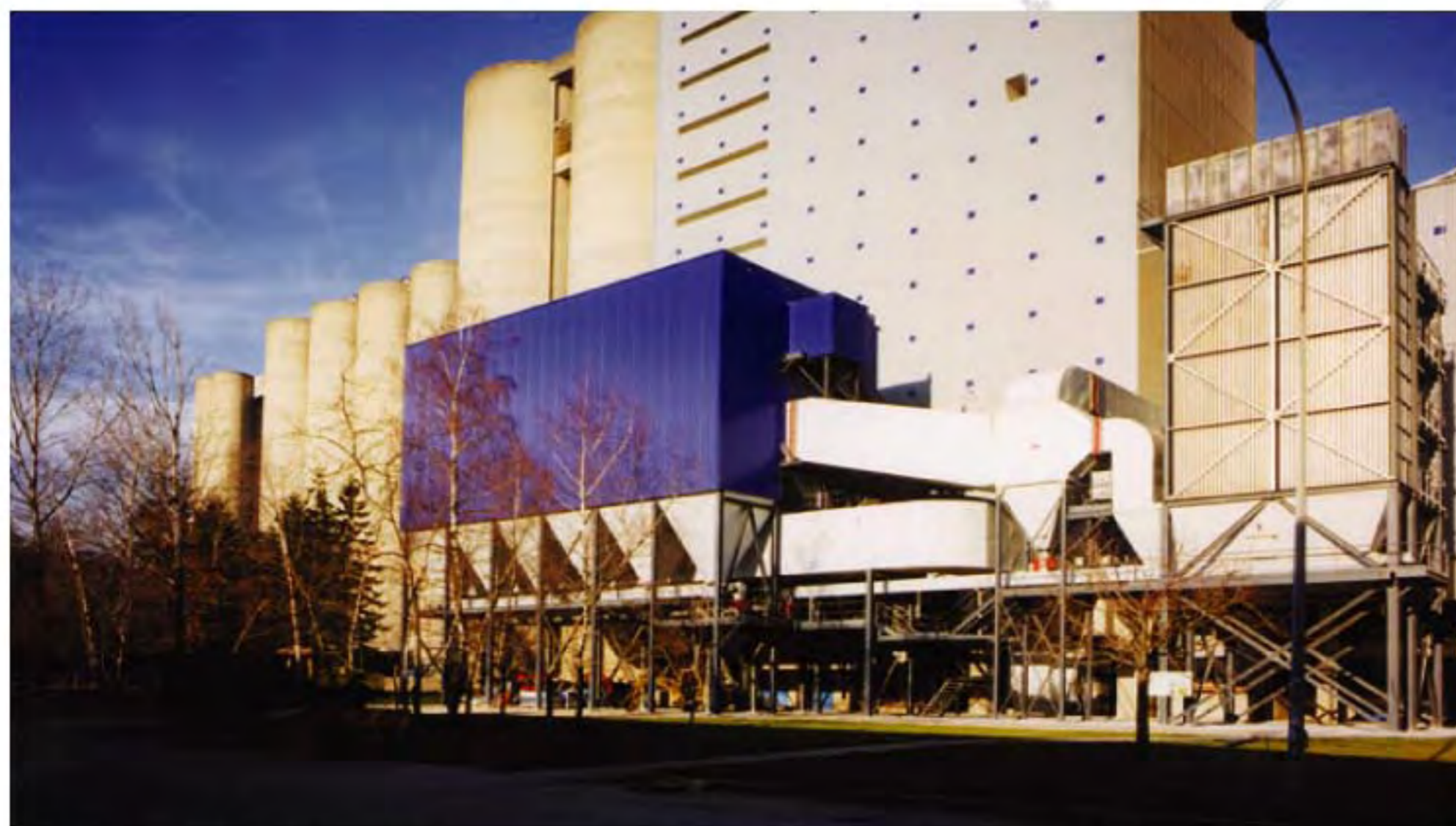
AAF Fabri-Pulse XLC and Forced Air Cooler installed in Holcim, France for Combined Clinker Cooler & Lepol Kiln dedusting.
