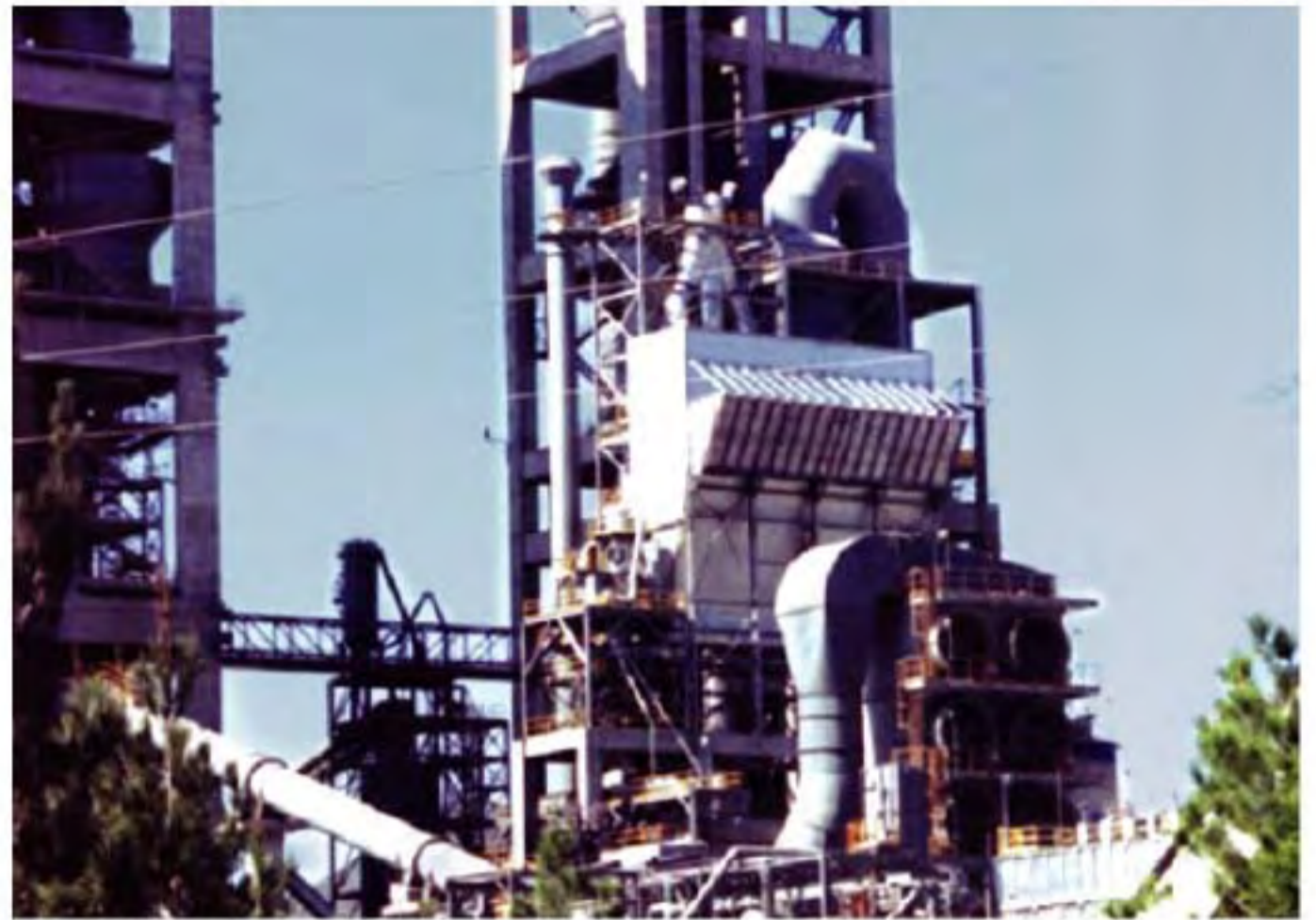
HOLCIM, Mexico. Fabri-Pulse Filter for Coal / Pekcoke Mill.
