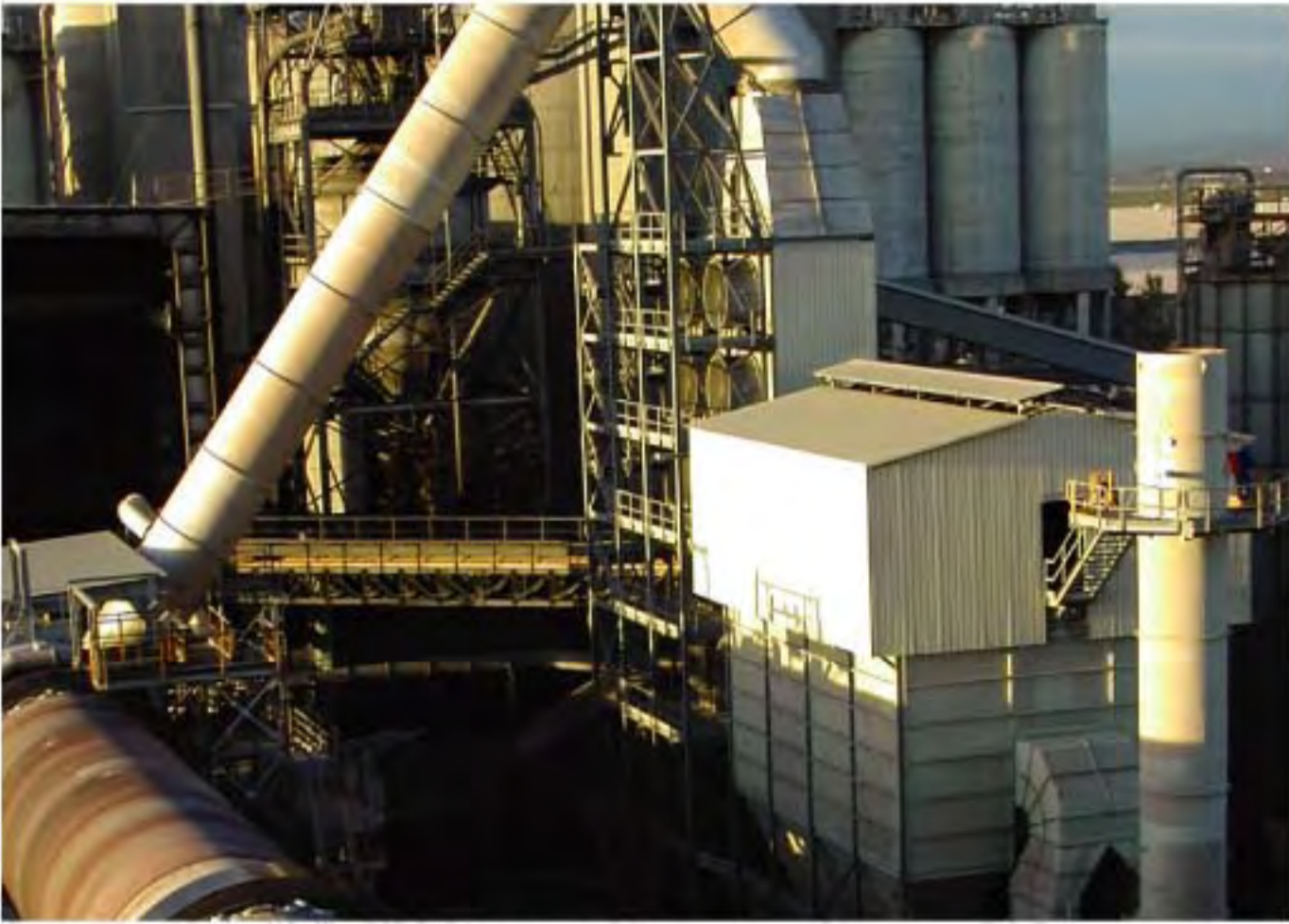
LAFARGE, Spain. Fabri-Pulse XLC Filter for Clinker Cooler.
