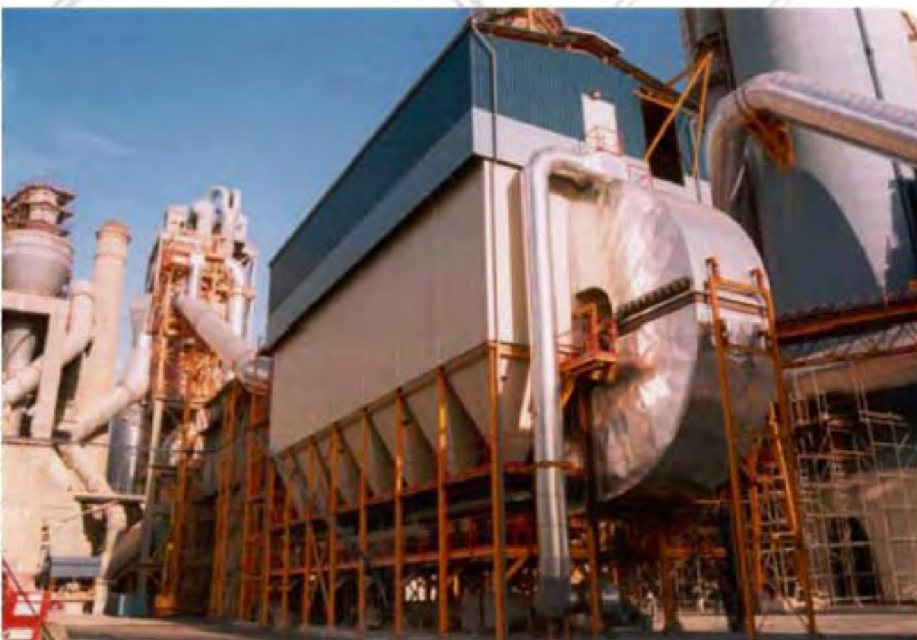
AAF fabric filter installed in Cimpor, Portugal for Kiln & Raw Mill dedusting.
